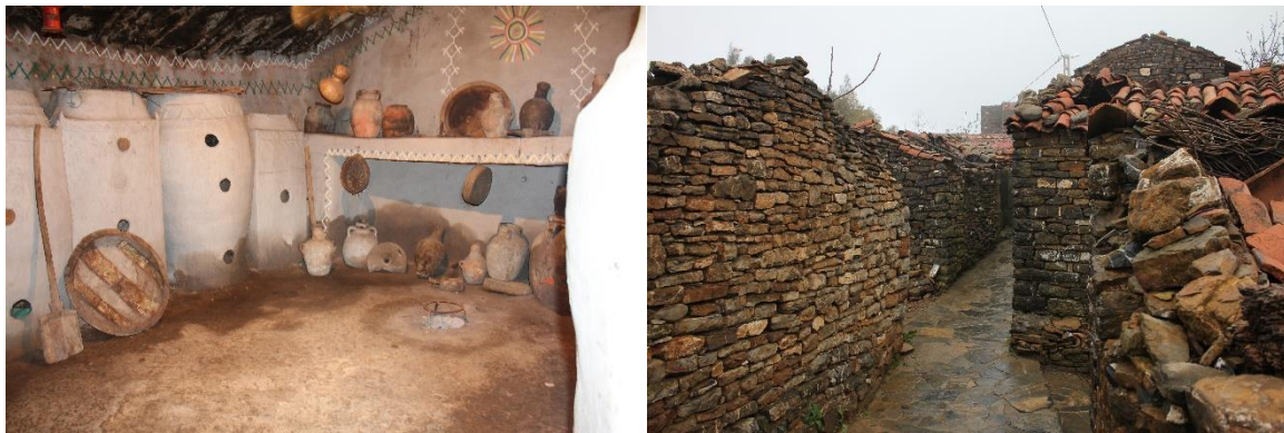
Photos 1 and 2. Showing the restoration of the house and alleyway siding, in Djebbla.
