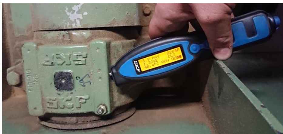
Figure 14. Difficulty accessing the bearing.
