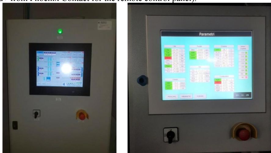
Fig. 7. Local engine control panel (left) and Remote control panel (right)
